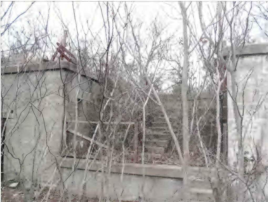
Figure 3.6. View looking north at emplacement #2, Battery Morris. Woody vegetation is growing in and around the stairs to the point where they are difficult to ascend and reach the gun platforms (Olmsted Center, January 2009).
